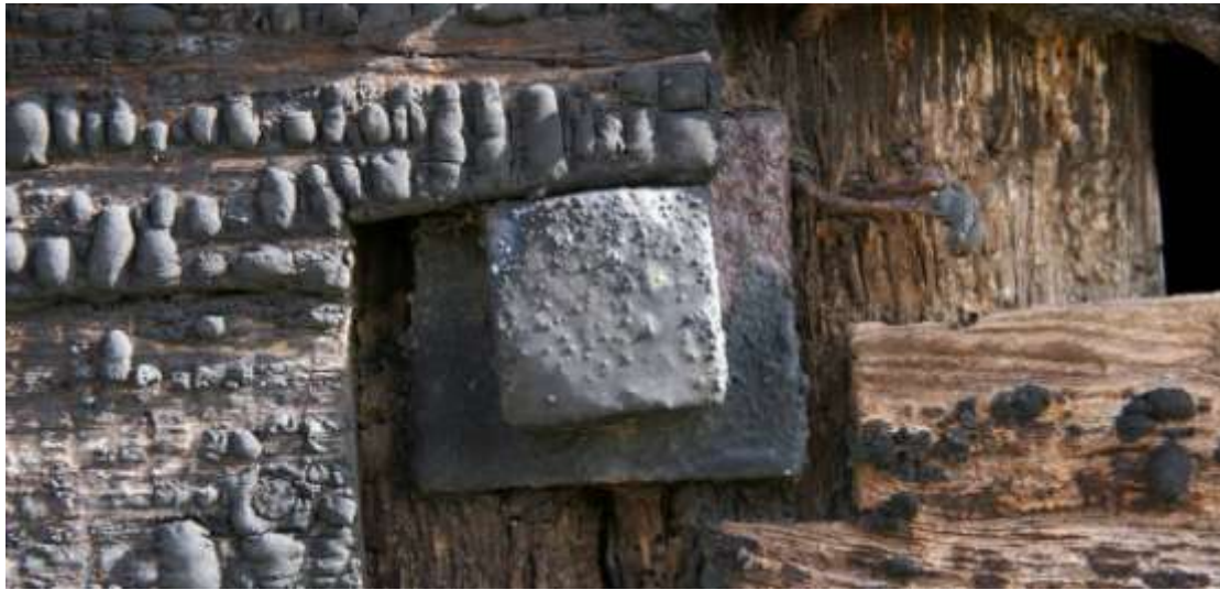
Head of a C19th / C20th bolt used to repair the barn.
